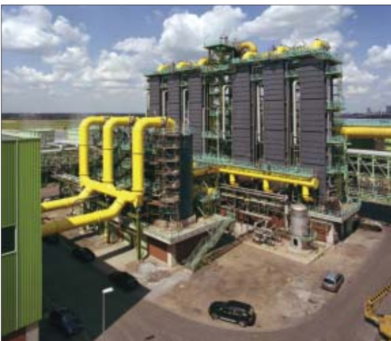
Fig. 2. Otto Simon specialises in consultancy and design/build services for the steel, water and energy industries.
